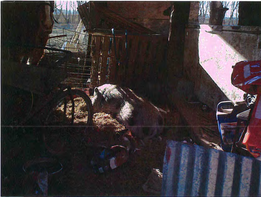
Date: 1/30/2015 Time: 3:42 P.M. Direction: west Photo by: S. Williams Exposure #: 027 Comments: animals are kept in dilapidated barn
