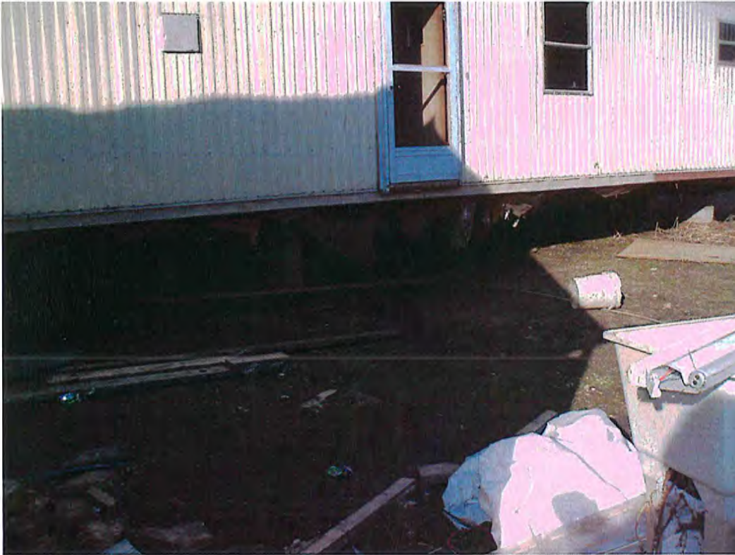
Date: 1/30/2015 Time: 3:05 P.M. Direction: northeast Photo by: S. Williams Exposure #: 005 Comments: materials from the underside of the mobile home have deteriorated
