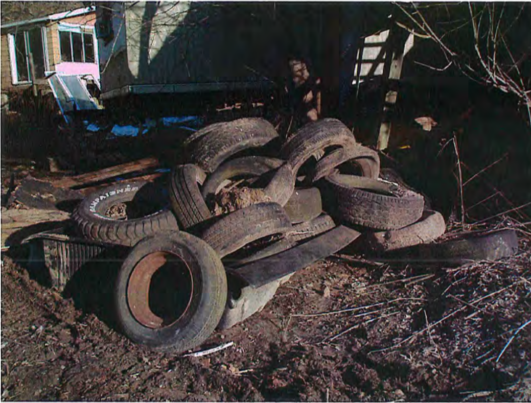
Date: 1/30/2015 Time: 3:33 P.M. Direction: southeast Photo by: S. Williams Exposure #: 019 Comments: tires and demolition debris
